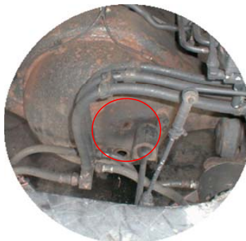
Corrosion hole [pit and dent]
